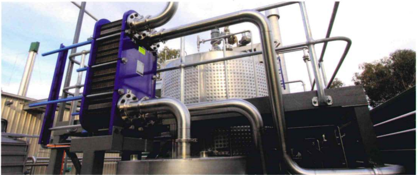
Licella commercial demonstration plant.
