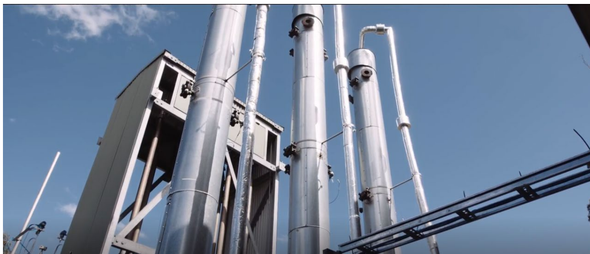
Figure 9: Cat-HTR™ commercial-scale reactors at the CS1 facility, Somersby, NSW
